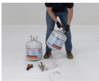
Shaking of A-side and B-side tanks
