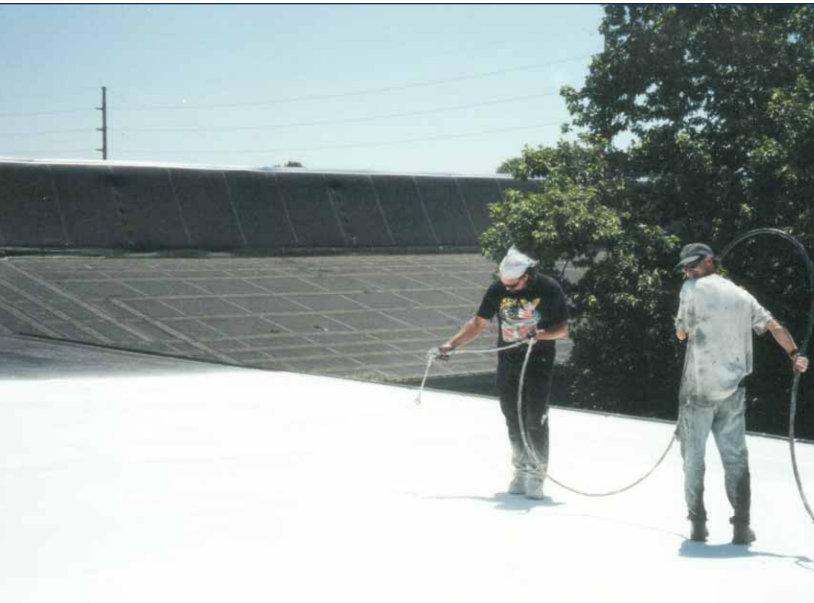
Acrylic coatings such as the one being sprayed on here can help extend the life of an old EPDM roof system (Photo courtesy of United Coatings.)
