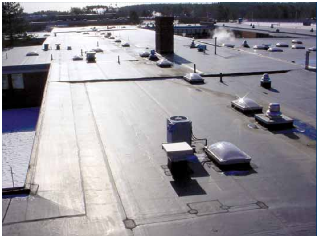
Finished view of Martinson Elementary School in Marshfield, Massachusetts. FleeceBACK applied directly over EPDM using FAST Adhesive made this roof as good as new.
