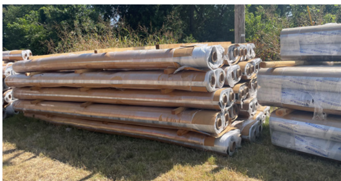
Improper jobsite storage of membrane
